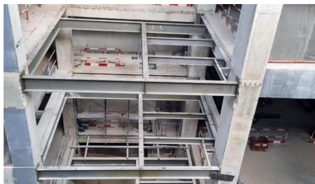
b) The steel frames are connected by anchors to the reinforced concrete structure
