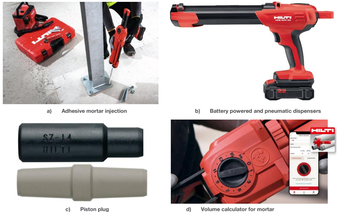
Fig. 8.11: Injection of adhesive mortar using automatic dispenser, piston plug and volume calculator app
