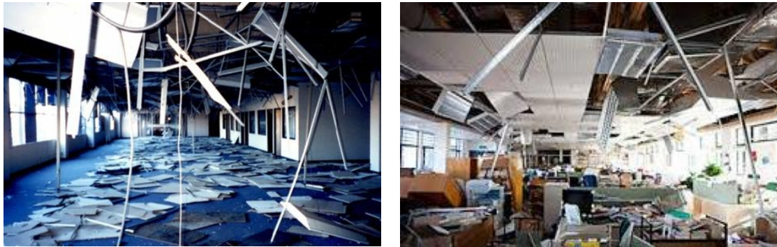
Fig. 9.8: Asset damage, production downtime for failure of non-structural connections
