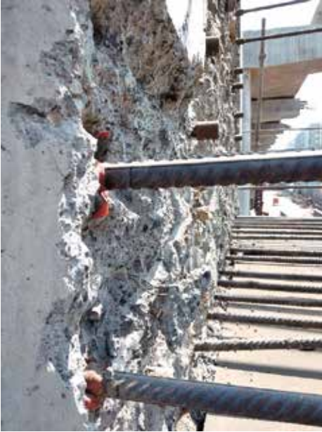
(a) Rebar in place of missing coupler
