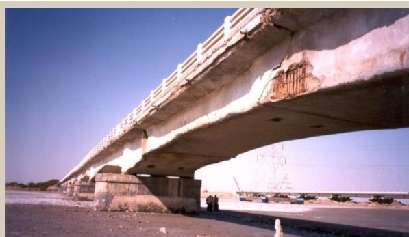
Fig. 4: Surajbari old bridge half joint in distress due to vertical and horizontal shaking
