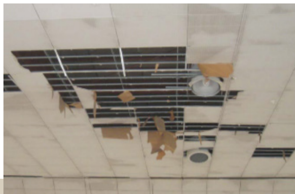
Fig. 3: Damaged ceiling in school gymnasium [10]
