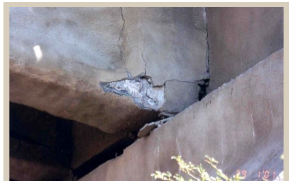
Fig. 2: Macchu Bridge superstructure pounded the dirt wall
