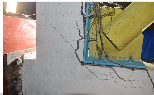
Fig. 2: Diagonal crack at beam-column joint
